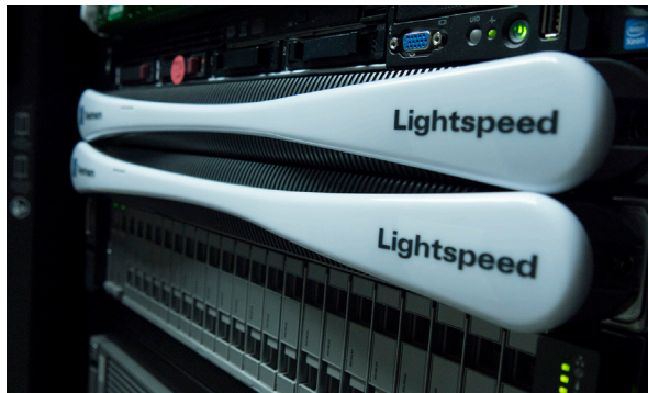
Telestream Lightspeed servers at work
